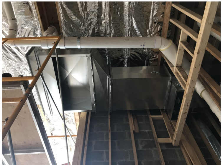
Ductwork - upper level ceiling
