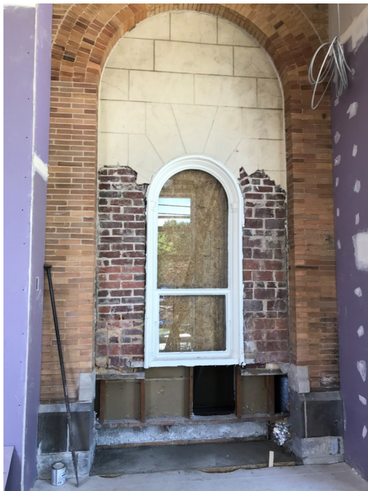
Demolition has begun: the view from the interior of the upper level of the new atrium.
